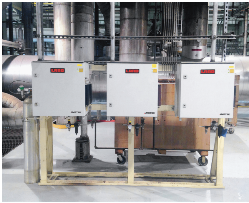
AMETEK Land millwatch analysers installed at the Merom power plant.
