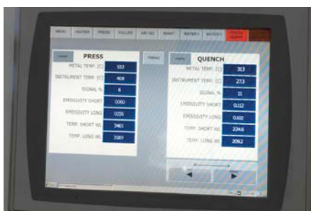
SPOT+ AL at the press exit and quench displayed on the customer's PLC
